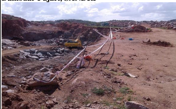
Above: Extensive blasting at the dam site now on going. Photo: Damodar Pujari, SANDRP
