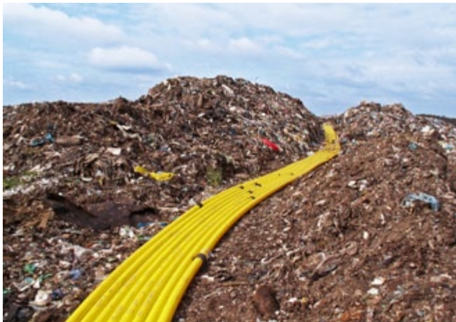
JI Mazurskie Landfill Gas Project in Poland, Courtesy of Mihai Brasoveanu
